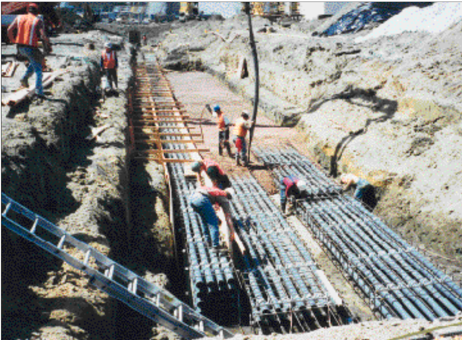
Brown and Caldwell managed installation of telephone and 12-kilovolt electrical duct banks in one of the San Francisco International Airport's main utility corridors as part of a 90-day fast-track relocation. The 52-foot-wide corridor also holds water, gas, sewer, industrial waste, and storm drain lines.
