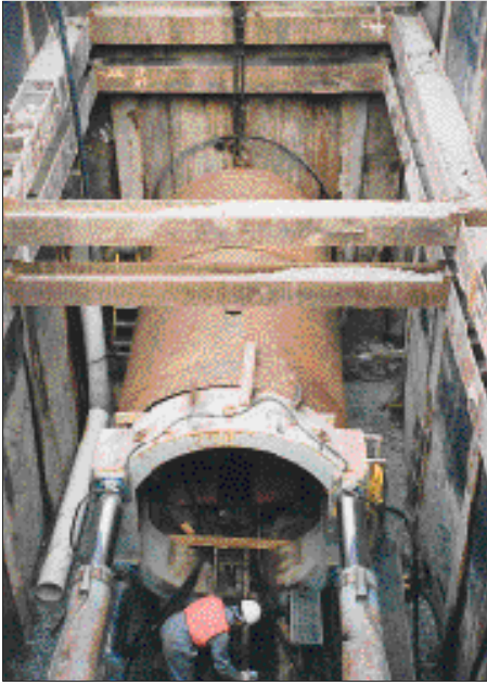
A jacking pit for boring an 84-inch-diameter reinforced concrete pipe casing under busy Highway 101. The pipe will house new water mains, electrical cables, and fiber optic cables. The work required continuous monitoring and surveying of settlement, along with close coordination with various agencies because it was done on restricted airport property surrounded by a state-regulated endangered species habitat.
