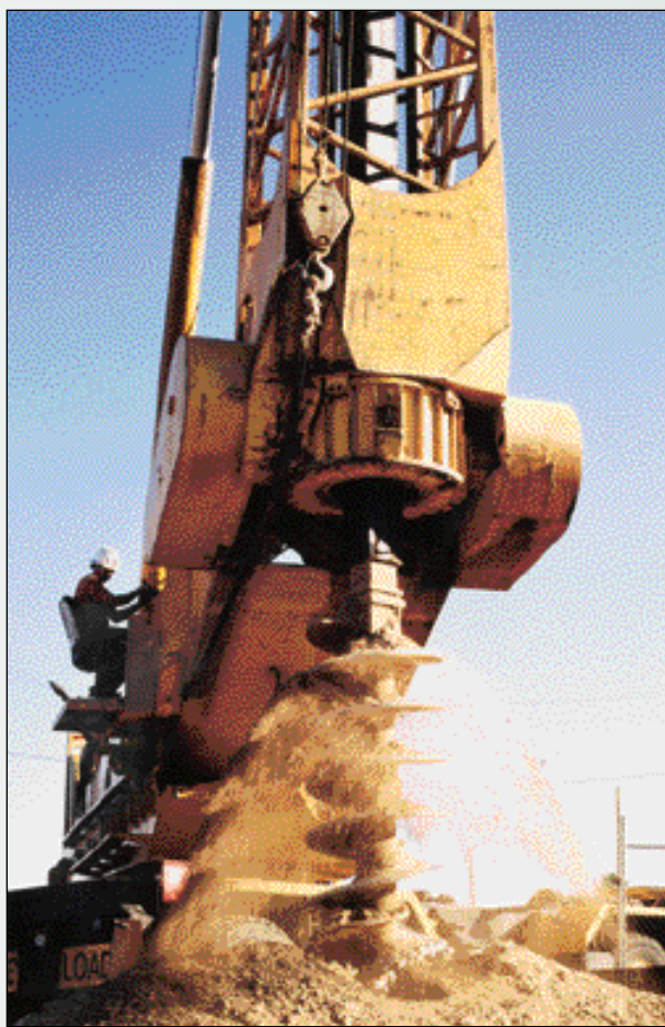
First-in-the-state use of a large-diameter flight auger to excavate contaminated soils at a former gasoline station saved time and money, allowing rapid regulatory case closure and sale of the property.
